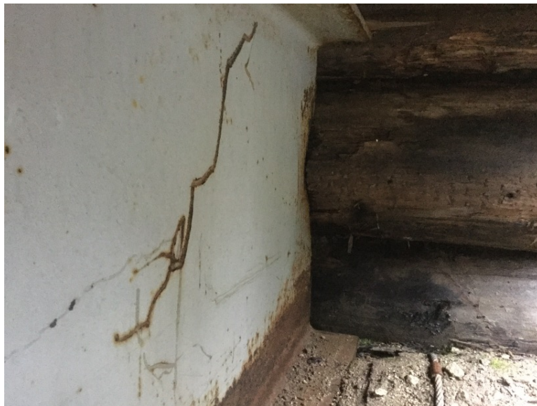
Minor web distortion
