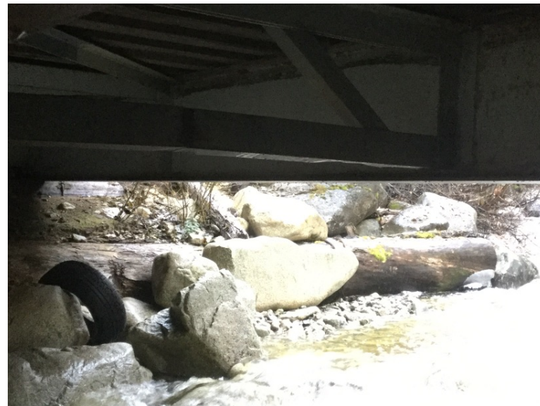
Bottom chord damage
